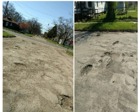
Potholes on Howden/Reynolds
