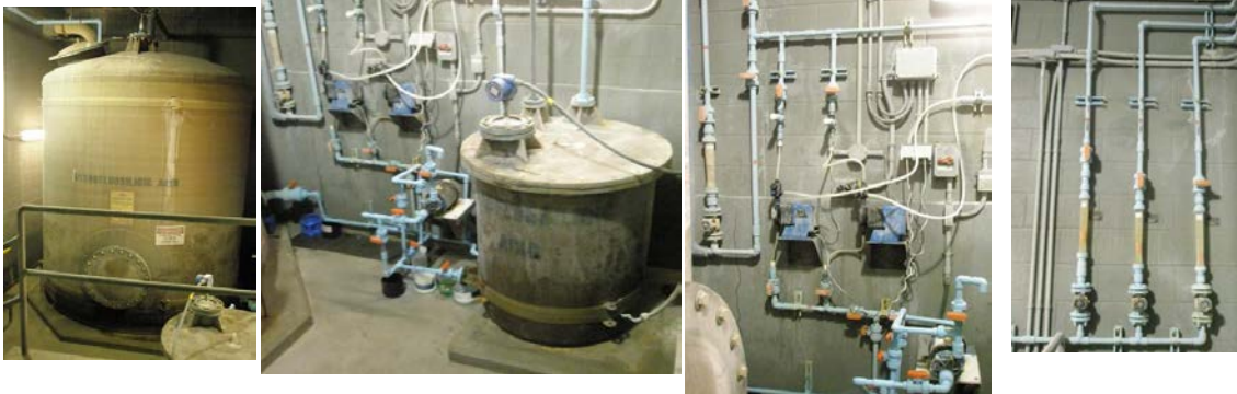
Fluoride: Bulk Tank, Day Tank & Transfer Piping, Feed Pump, Feed Points
