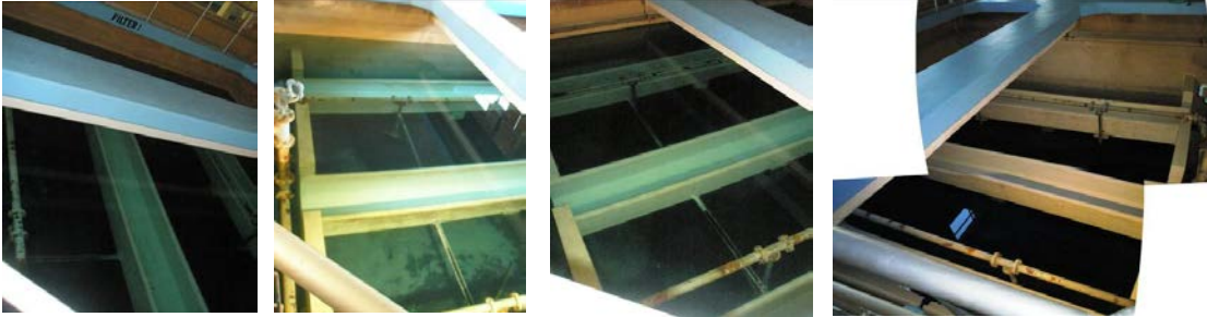
Filter Nos. 5, 6, 7, and 8
