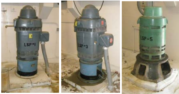
Low Service Pump Nos. 1, 3, and 5
