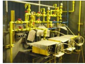
Chlorine Feed Pumps 1,2,3 (Top); 4,5,6 (Right) ; 7,8,9 (Left)
