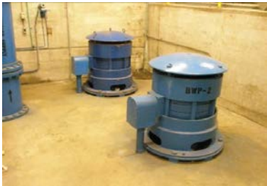
Backwash Pump No. 1 & No. 2
