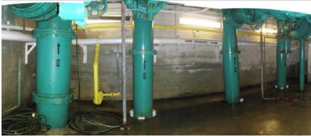
Low Service Sub Level Piping (1, 3, 5)
