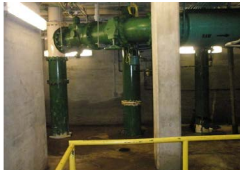
Low Service Sub Level Piping (4, 6, 2)
