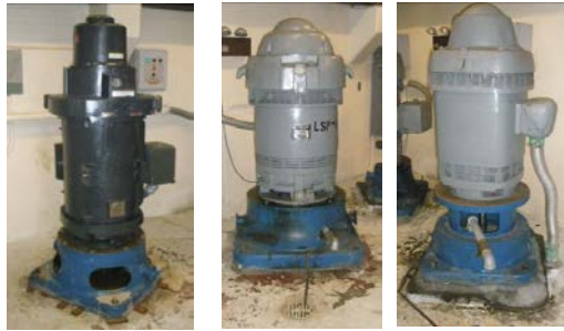
Low Service Pump Nos. 4, 6, and 2
