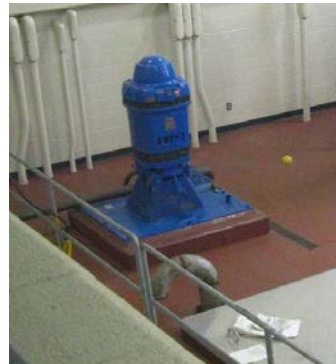
Backwash Pump No. 3
